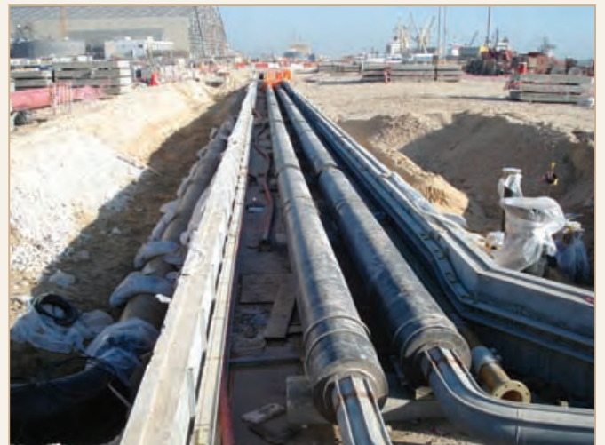
Sulfur pipelines with SEEHT system arriving at berth area
