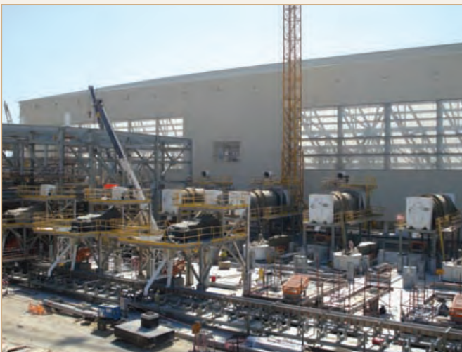
Granulators being installed
